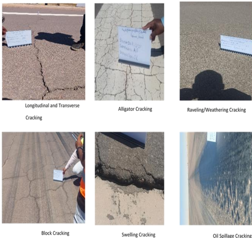
Figure (4). Several types of distress on the runway fixable surface on RY 13/31
